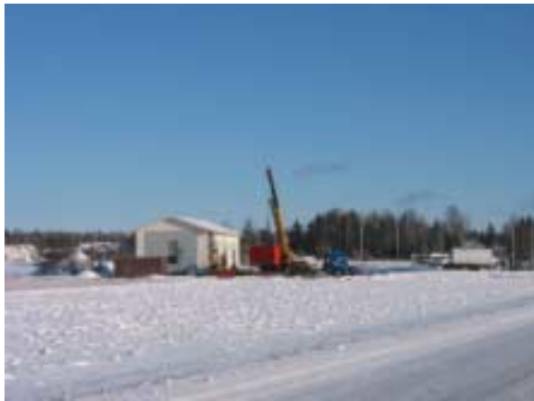
Left: The construction of a district heating plant for wood chips is an important step in converting all municipal buildings to biomass heating Vörå, Finland.
