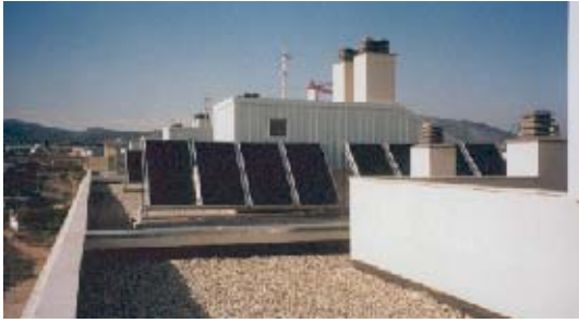
Solar heating system, Vilanova
