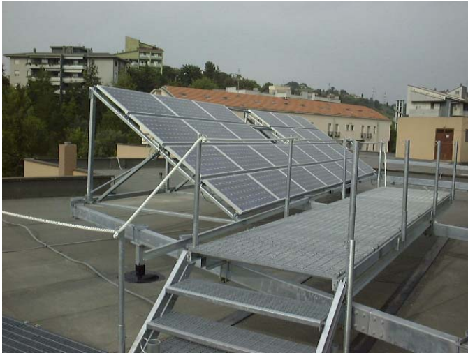
Picture 1: Realized PV installation
