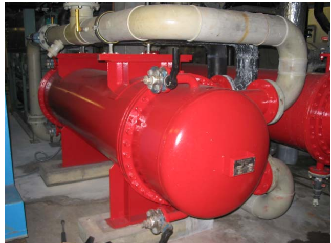
Heat recovery unit
