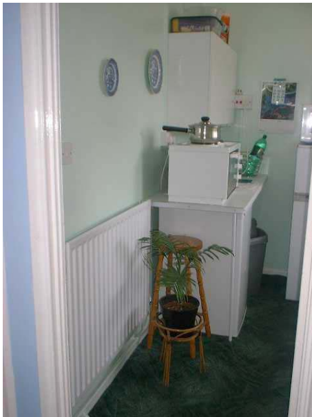
GSHP heated radiator
