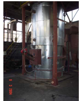
The Wood briquette boiler
