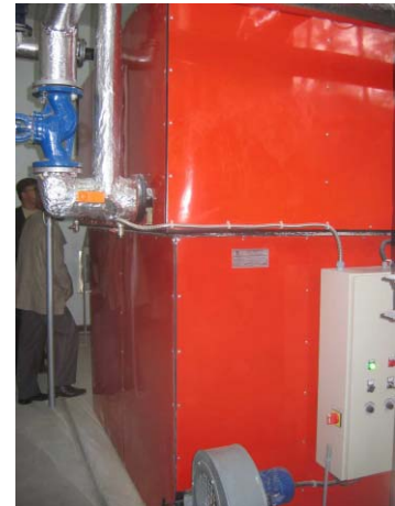
Wood chips boiler
