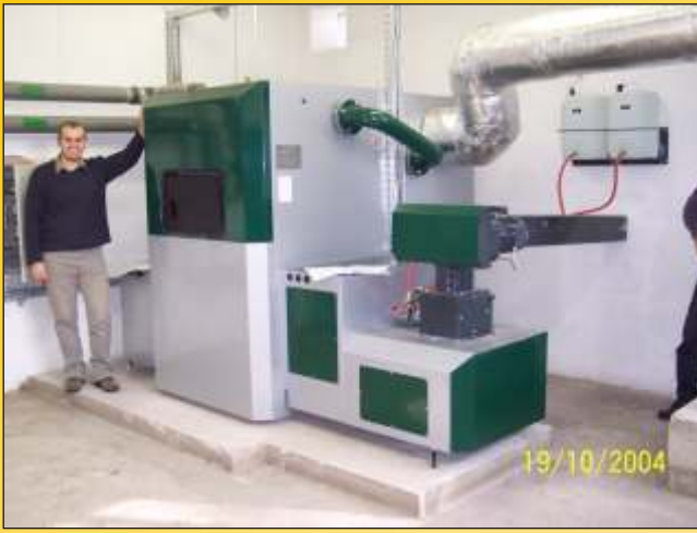
Boiler room after reconstruction
