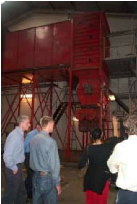
Inside the plant at Sätenergi
